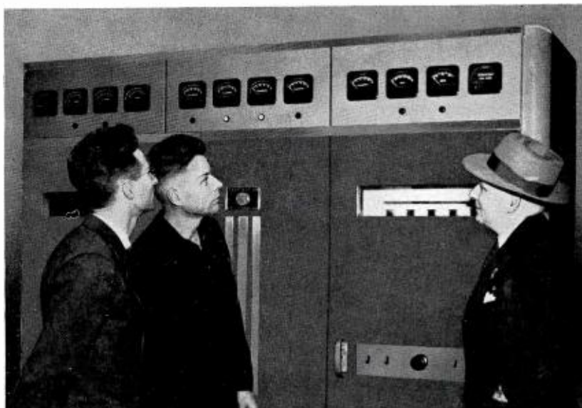
Inspecting WOPI-FM's newly installed BTF-3B Transmitter. Left to right: P. G. Walters, RCA Southeastern Regional Office; W. E. Tucker, RCA Engineer; W. A. Wilson, President and General Manager, WOPI and WOPI-FM.
