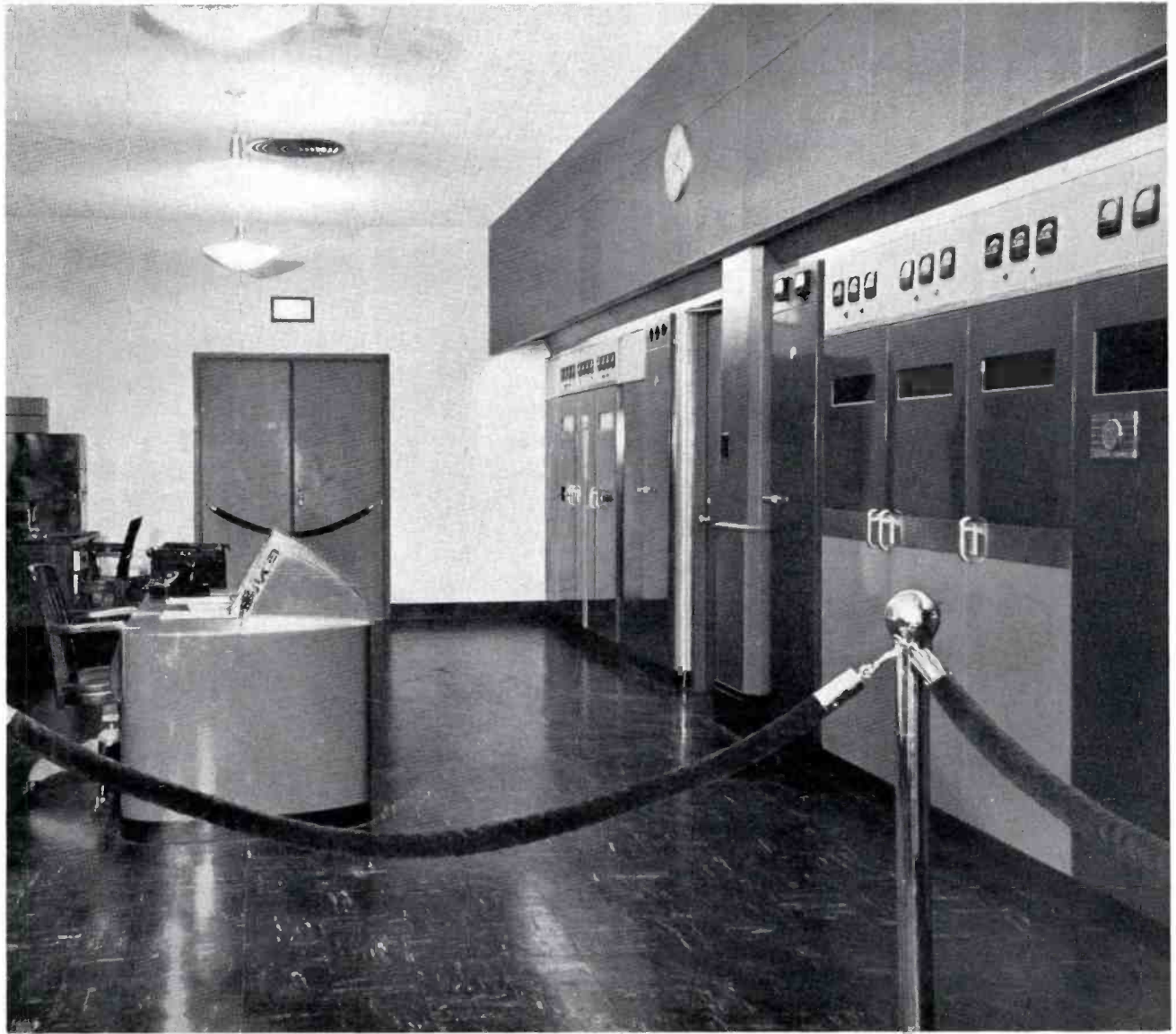
FIG. 2. The BTF-3C FM Transmitter and the TT-5A Television Transmitter are located in a first floor wing of the hotel.
