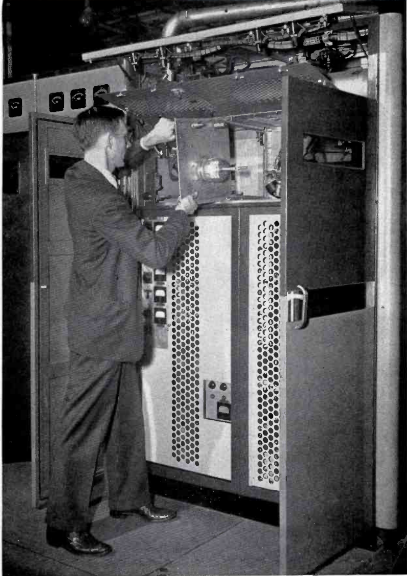
FIG. 1. The 8D21 tubes in the TT-5A transmitter are mounted on "tube plates" which can be easily removed whenever it is necessary to make a quick tube change.
