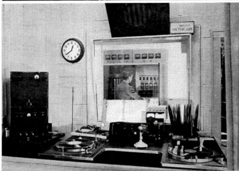
View of the studio control room of WOPI-FM. Through the control room observation window can be seen the power panel of the transmitter.
